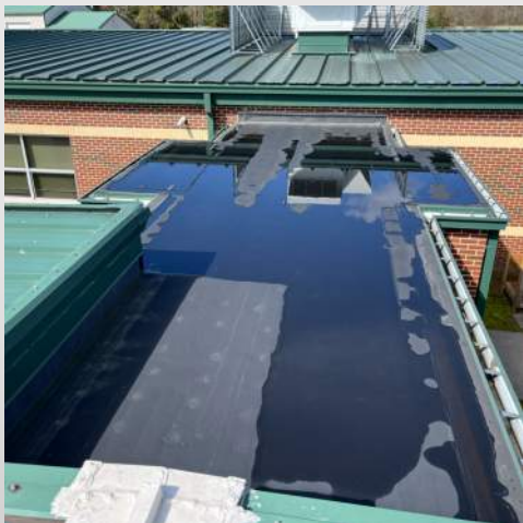
Roof Material Degradation, Ponding Water, Roof Drains, Debris & Algae Growth
