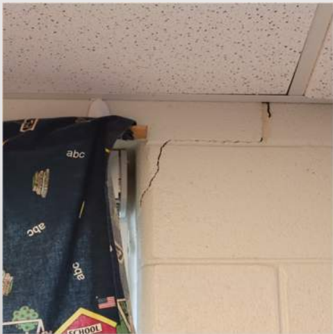
Masonry Cracking, Movement, Delamination & Mortar Deterioration
