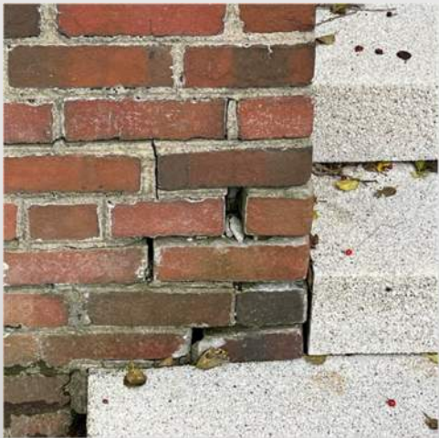
Masonry Façade Cracking, Movement, Delamination, & Mortar Deterioration
