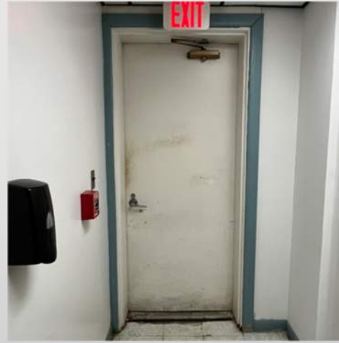
Exit Door Hardware
