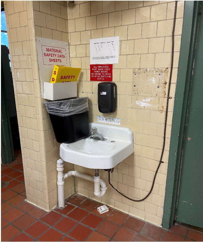
PHOTO K.2 THE HAND SINK FAUCET NEEDS TO BE REPLACED AND A TOWEL DISPENSER NEEDS TO BE INSTALLED.
