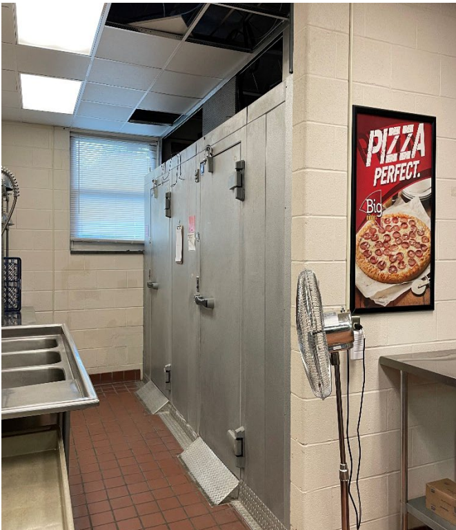
PHOTO K.3 THERE ARE STEEP RAMPS UP TO THE WALK-INS AND THERE ARE MANY CEILING TILES AND TRIM MISSING.
