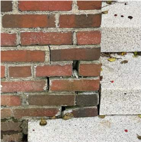
Masonry Façade Cracking, Movement, Delamination, & Mortar Deterioration
