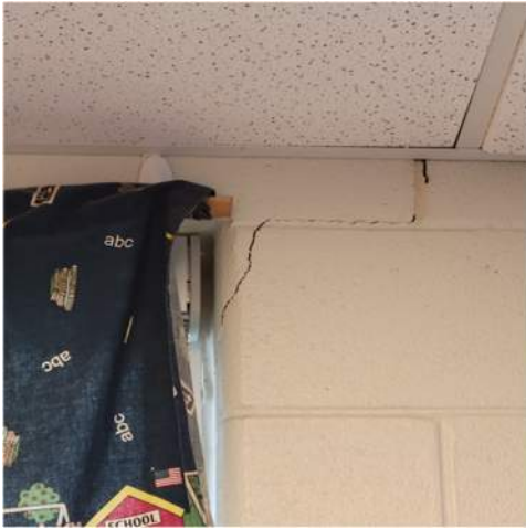
Masonry Cracking, Movement, Delamination, & Mortar Deterioration
