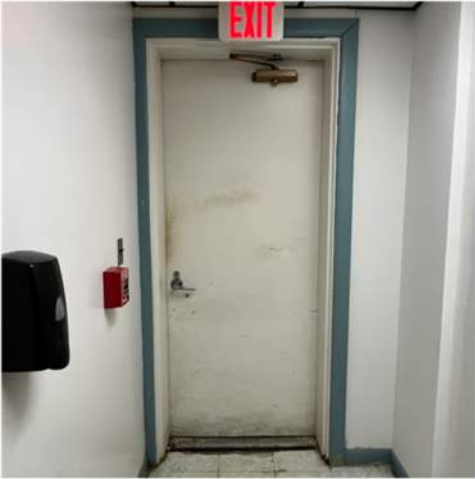
Exit Door Hardware
